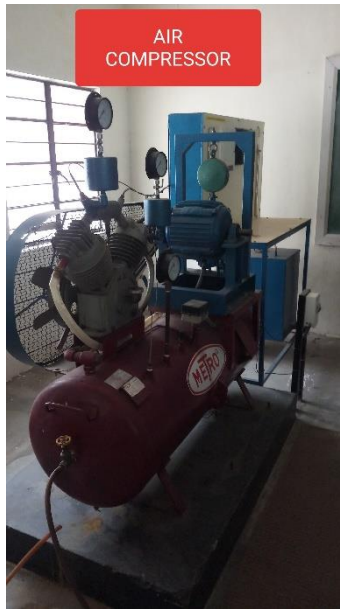
Fig. 3 Air compressor equipment
